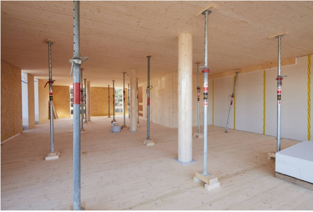
During the curing of the casting resin, the floor slabs must be additionally supported
